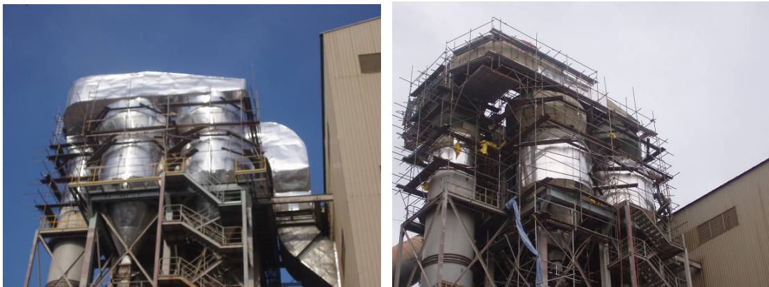
Insulation of Raw Mill Cyclone
